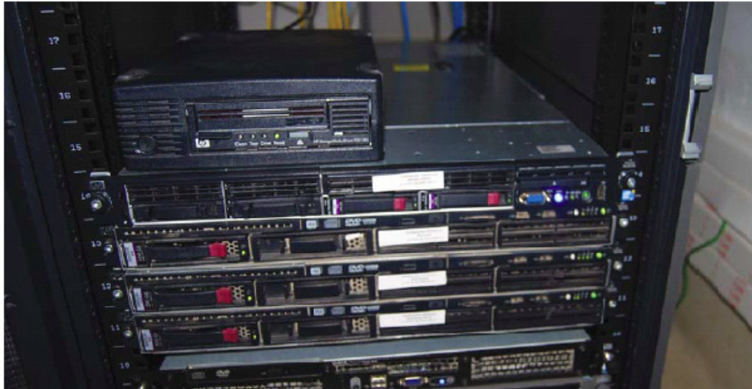
New servers installed at the CISM.
